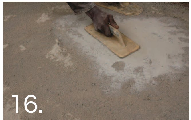
Wood float the Colour Hardener into the surface. If it is necessary to add water; dip the plastic float in a bucket of water; DO NOT use a block brush to flick water onto the screed.
