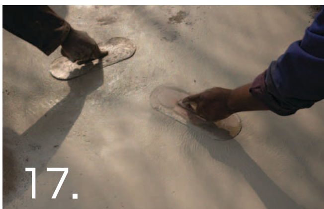
Apply a second dusting of Colour Hardener at a rate of 3kg/ m 2 . Allow to soak in the moisture from the screed, then plastic float and steel trowel.
