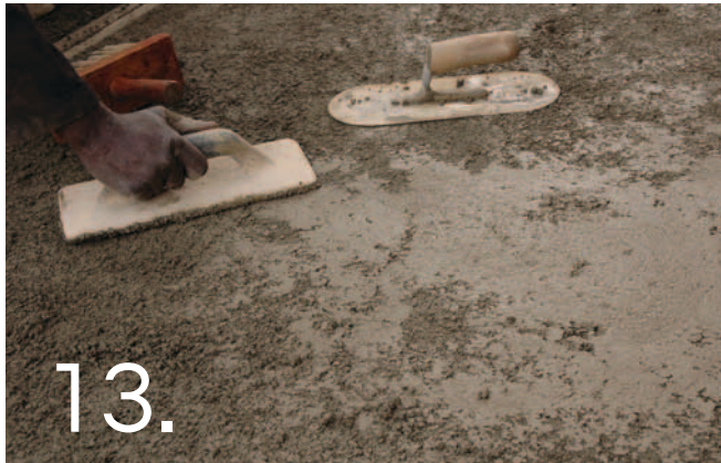
Wood float screed. If additional water is required, wet the plastic float only; do not spray the screed directly with water.
