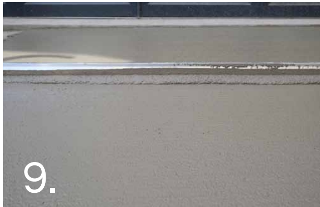
9. Avoid dry joints by completing the application to the entire control joint panel in a continuous operation. Repeat entire process for each panel. Note: No panels should be left partially filled as cracks will appear when the new Exposed Aggregate is applied at a later stage.
