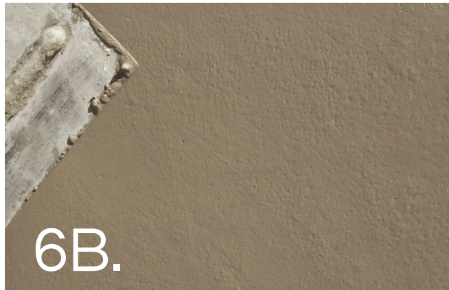
Smooth Finish (3mm) | Finish using a steel float, being careful not to "burn" by over-trowelling.
