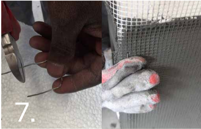
Keep the mesh firmly in place using industrial staples or pieces of thick U-shaped wire.
