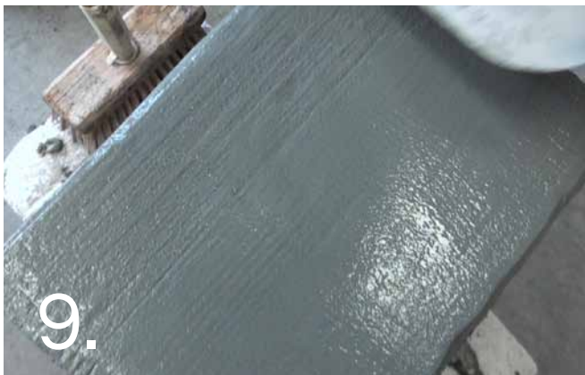
While the final coat is still damp, lightly wet the surface and follow with a steel trowel to achieve a smooth final finish. Allow to dry completely. The base / one side may need to be completed separately.
