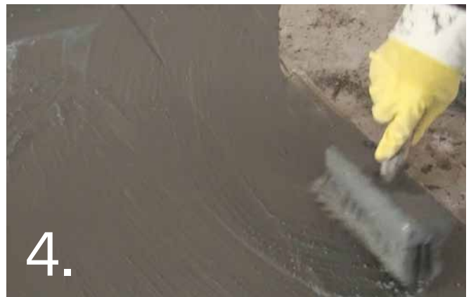
4. Apply PrimerCote slurry to small sections at a time, cover with screed mix and repeat. Do not apply too thin and do not allow to dry prior to covering with new screed mix. Immediately place screed mix onto wet slurry.
