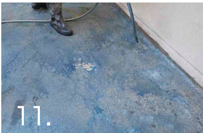
11. Although the retarder is blue in colour, a second person can assist the person spraying, ensuring the whole floor is sprayed evenly so as to obtain an even aggregate exposure. The retarder must be shaken before use and frequently agitated during use. Spraying is preferably done using an airless spray gun with a medium tip nozzle between 1.2mm and 2.5mm. The wet Exposed Aggregate must have no bleed water on it prior to the application of the retarder.
