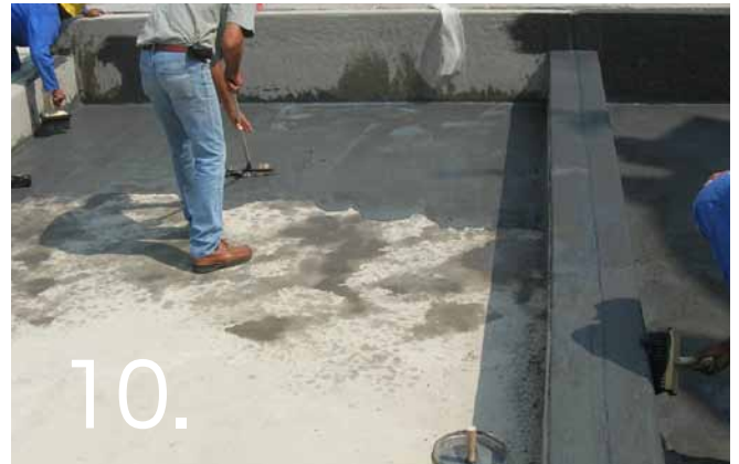
10. Soft brooms may be used to apply the MatCrete for larger areas.
