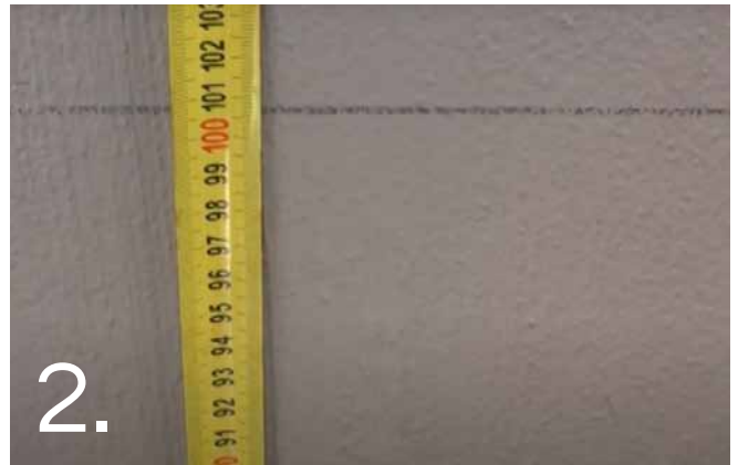
Strike a level chalk line approximately 1 meter from the finished ground level.
