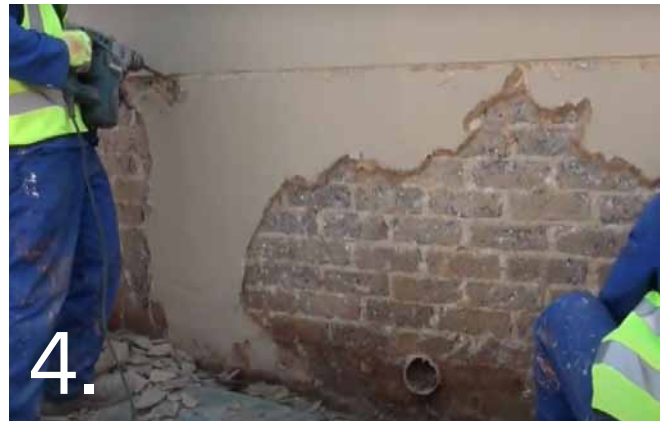
Remove all plaster down to brick level and clean thoroughly to ensure that no dust remains.
