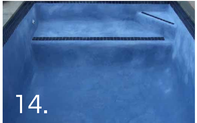
14. Filling of the pool can commence \pm 6 to 8 hours after plastering has been completed depending on ambient temperatures & relative humidity where plastering has been completed early afternoon. Where this is not the case & the plastering is completed late afternoon or early evening it is recommended that the filling process commences the morning following the application.
