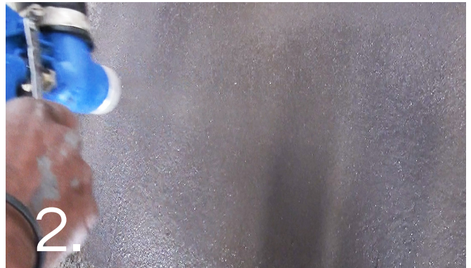
2. Spray apply the first coat with a 5mm hopper gun nozzle at a high pressure and allow to dry. Then dampen with water and apply the second coat as per first coat. Once completely dry, dampen with water again and use a mechanical blower or broom to clean off the area free of unbonded material and dust. Then use a coarse broom to remove any overspray.
