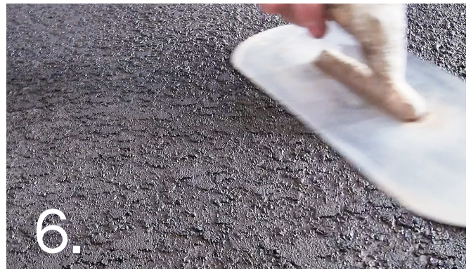
6. ..."knock down" the sprayed mortar with a 300mm rounded steel trowel. Once completely dry, use a mechanical blower or broom to clean off the area free of un-bonded material and dust. Then use a coarse broom to remove any overspray. Then continue with the curing and sealing process.
