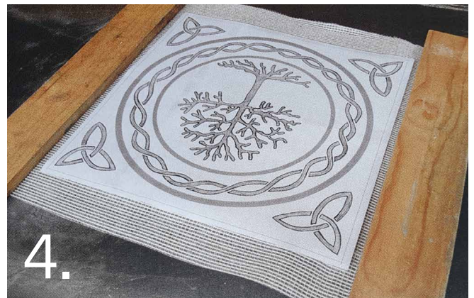
4. Place pieces of wood on the side of the CemLam. This will act as a guide to ensure the correct thickness of the slab. It will also help create a level surface.
