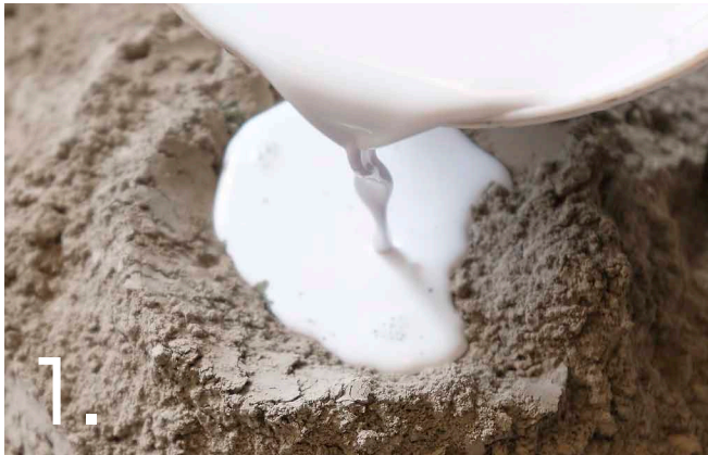
1. In a suitable container, combine 1 volume of mixing liquid (1 volume FlexBond with 4 volumes water), and 2 volumes of SculptCrete powder.
