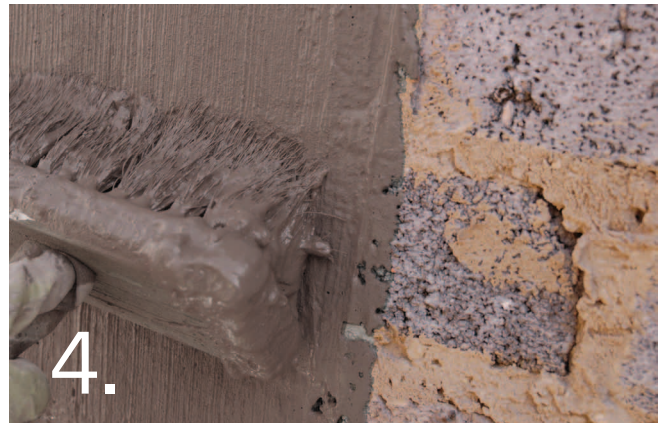
4. Mix 3 volumes of CemWash first coat grey with 1 volume of clean water. Mix to a paste, then add further volume of water. Mix to a creamy slurry. Apply with a block brush. Clean splashes and over-brushing at the end of each day. Cure by wetting with clean water 3 times during the next day. Leave to dry.
