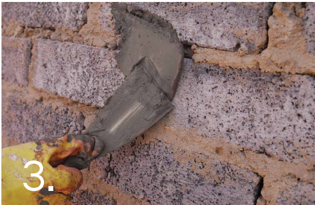
3. Prepare a paste comprising 3 volumes of CemWash and 1 volume water. Fill large holes using this paste. Leave to dry for 1 day. Cure by wetting with water 3 times during the next day.
