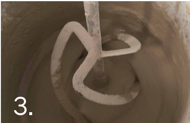
In a suitable container combine 3 volumes CemWash first coat grey with 1 volume of the Mixing Liquid. Mix to a paste. Add 1 further volume of the Mixing Liquid. Mix to a creamy slurry.
