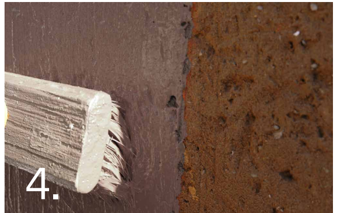
Apply the CemWash first coat grey using a block brush. Clean slashes or over-brushing at the end of each day. Cure by wetting with clean water 3 times during the next day. Leave to dry.
